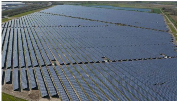
PUBLIC SOLAR PV
